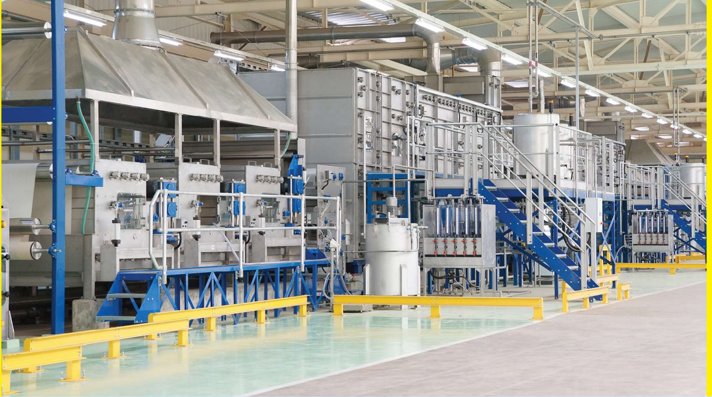
CONTINUOUS SCOURING BLEACHING RANGE
